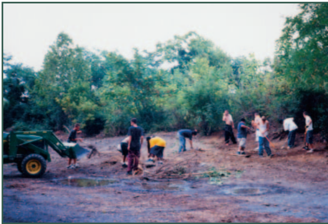
Youths from TresslerCare Wilderness Center programs contributed more than 1,200 hours of community service last year to the Capital Area Greenbelt Association in Harrisburg. Here, students from the center work on clearing ground as they continue efforts to conclude the greenbelt project, which was begun 102 years ago.
