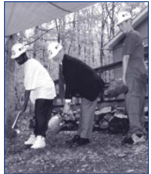
Breaking ground for the Wilderness Center's expansion are, from left to right, current student Jason Kissinger, Wilderness Center Executive Director George Eckenrode, and Hosea Twiggs of Philadelphia, a former student and recent high-school graduate.
